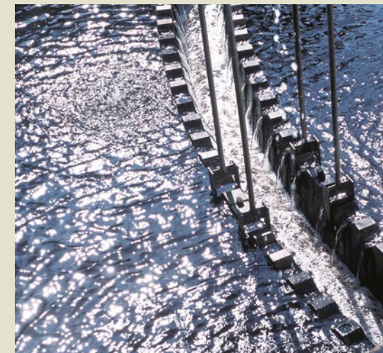
Part of the wastewater treatment plant in Krefeld – Uerdingen
